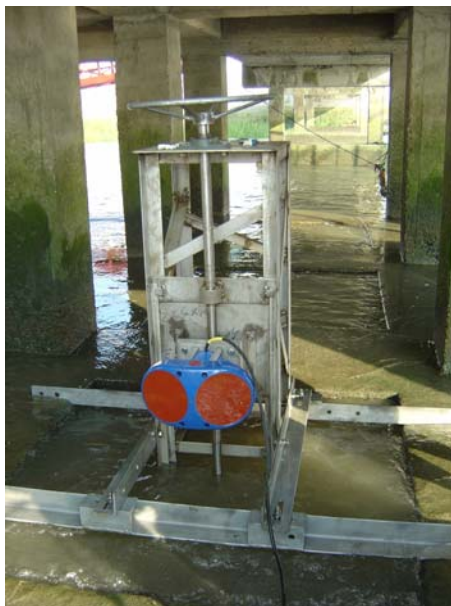
Figure 3 A 300 kHz H-ADCP at Songpu Bridge hydrology station in Huangpu River, Shanghai, China
